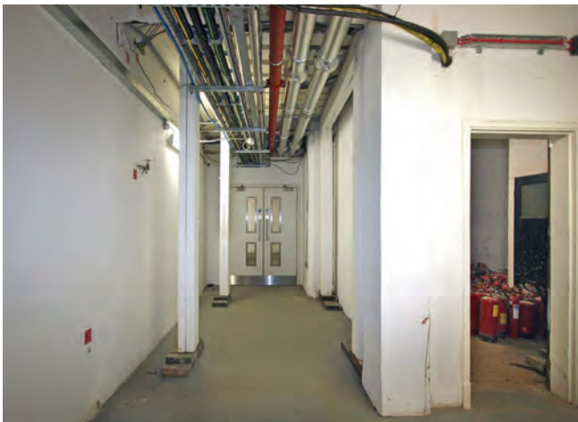
Wartime timber strutting under Quadrant Arcade miraculously surviving through seven decades of refurbishment. Four stanchions formed of doubled up timber boards resting on large timber wedges bolster up a small section of arcade floor. Photo Nick Catford
